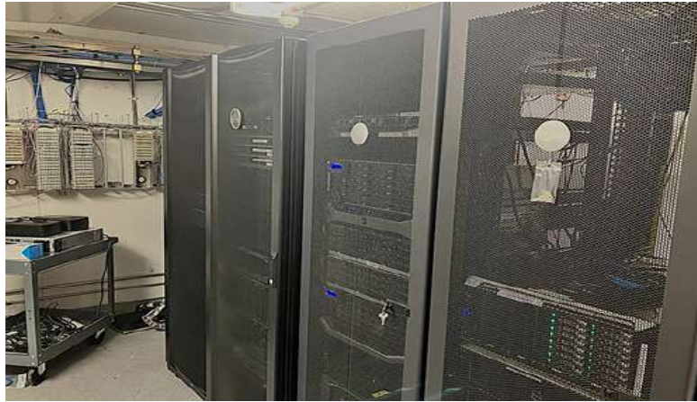
Telecommunications room of the Neurosurgery Research
